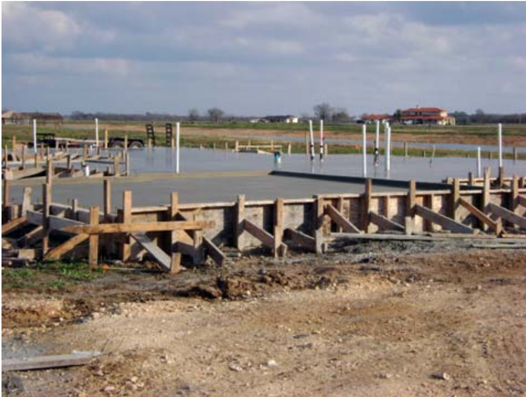
Above: Another foundation is poured just in time for an early Christmas present.
